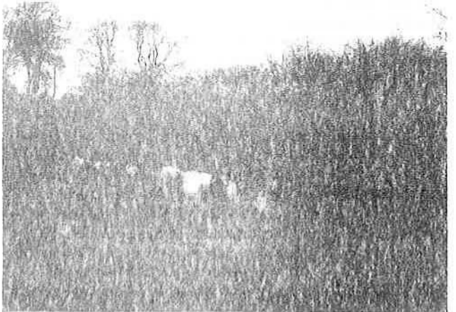
e) An offside embankment with low freeboard, vulnerable to stock damage – Macclesfield Canal. (PFP)
