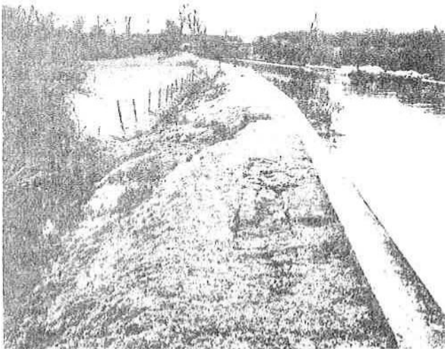
Plate 12.8 This embankment on the Grand Union Canal has a history of persistent leakage problems (PFP)
