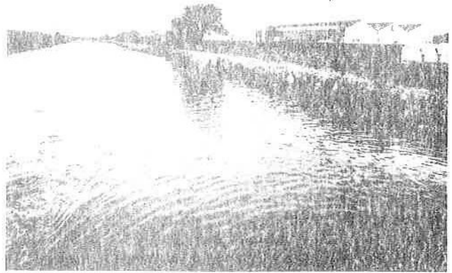
d) Advanced erosion of a towpath threatening the foundations of a boundary wall – Sheffield and South Yorkshire Navigation. (PFP)
