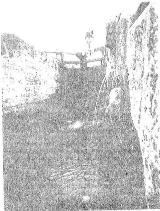
Plate 12.9 Water pouring out from cavities behind a lock chamber wall — Llangollen Branch of the Shropshire Union Canal (PFP)
