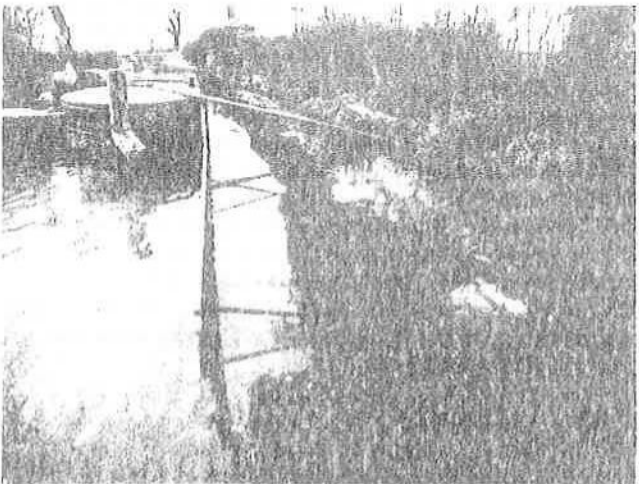
b) A towpath embankment with virtually no freeboard now being re-protected and back filled – Grand Union Canal. (PFP)
