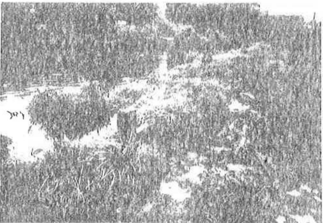
c) Temporary repair to an offside embankment, only the plank prevents overtopping – Staffordshire and Worcestershire Canal (PFP)
