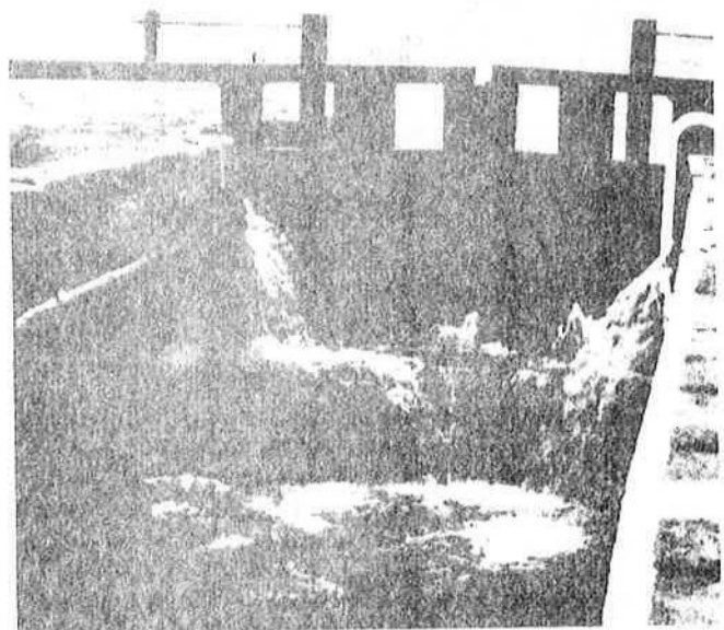
Plate 12.10 Leakage between gate heel posts and chamber quoins, etc. — Leeds and Liverpool Canal (PFP)
