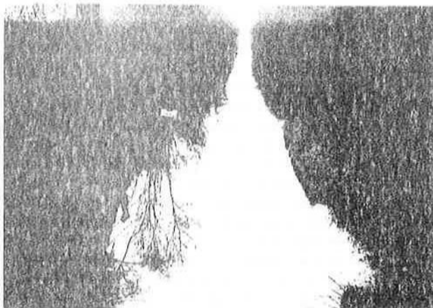
Plate 12.7 Extensive erosion following failure of dry-stone walling on the towpath side – Shropshire Union Canal (PFP)
