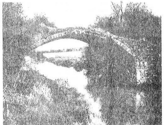
Plate 12.12 Derelict accommodation bridge -- Oxford Canal (South) (PFP)
