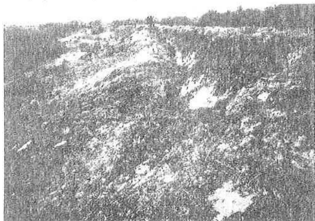
Plate 12.15 Embankment slip at New Bradwell on the Grand Union Canal, January 1975. (PFP)
